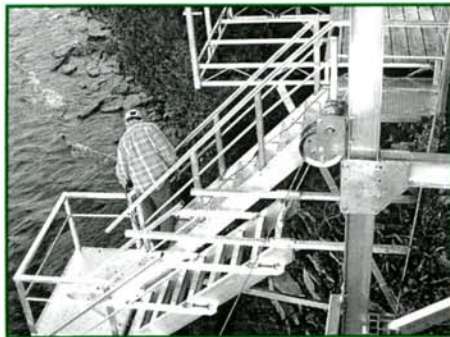
HD STAIRWAY • DOWN TO 8' X 16' DOCK • 25' FROM GROUND LEVEL TO WATER • STAIRS HINGE AND LIFT AND THE DOCK LIFTS ALSO I BEAM FRAME AND HINGE • DRILLED PINNED TO ROCK • LIFTS EASILY WITH HAND WINCH FOR WINTER STORAGE Sackets Harbor
