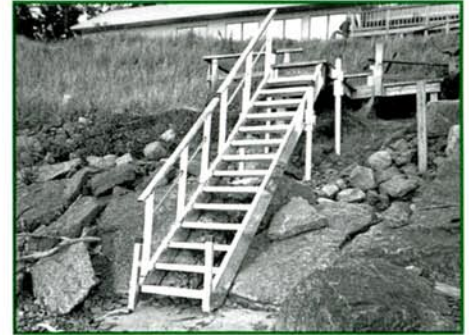
HEAVY DUTY TWO PIECE STAIRWAY WITH RAILING DRILLED & PINNED TO ROCK • LOWER SECTION REMOVABLE TO PREVENT ICE DAMAGE Lake Ontario
